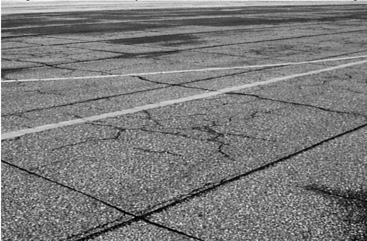
Reflection Cracks Asphalt overlay over concrete
