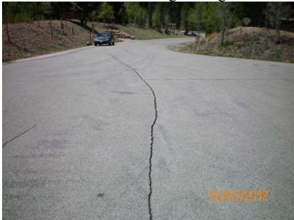
Longitudinal Cracks on Peerless Drive
