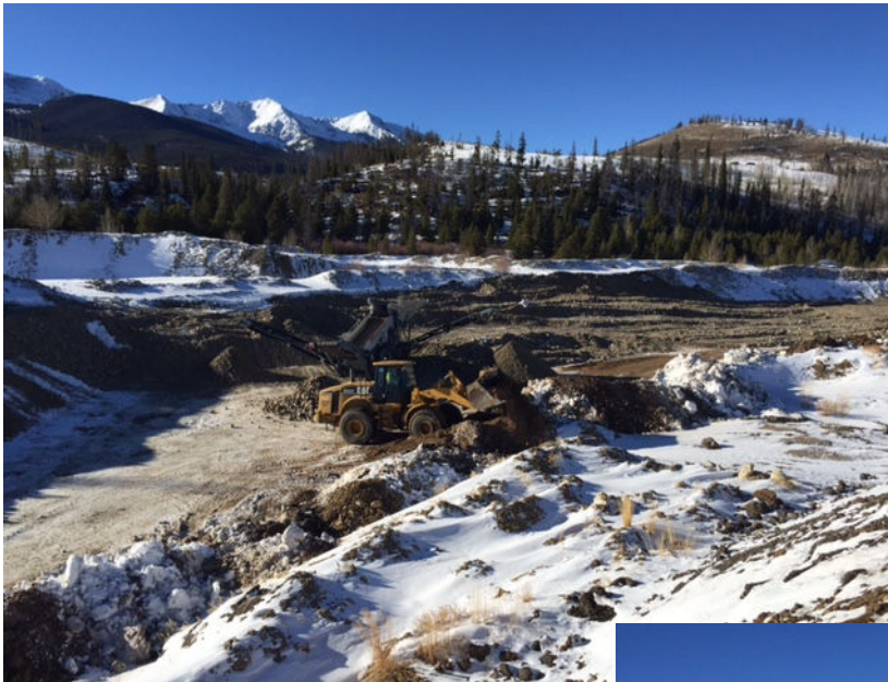
Tezak crew beginning to process on site dredge materials for use in the temporary channel.
