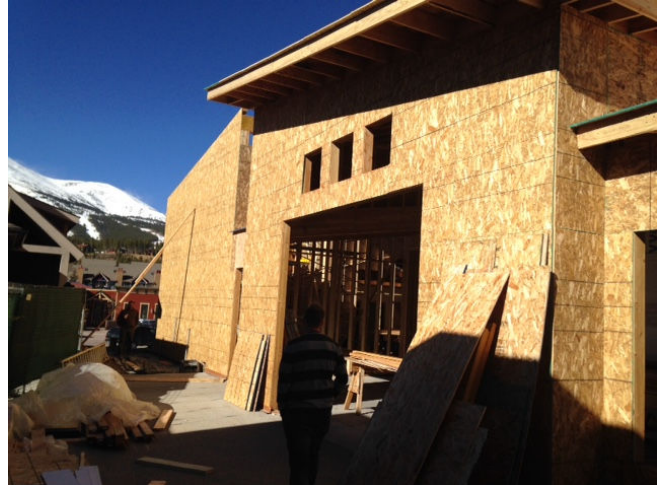
Wall framing for the garage door that opens to the plaza connecting to Ceramics and the Hot Shop.
