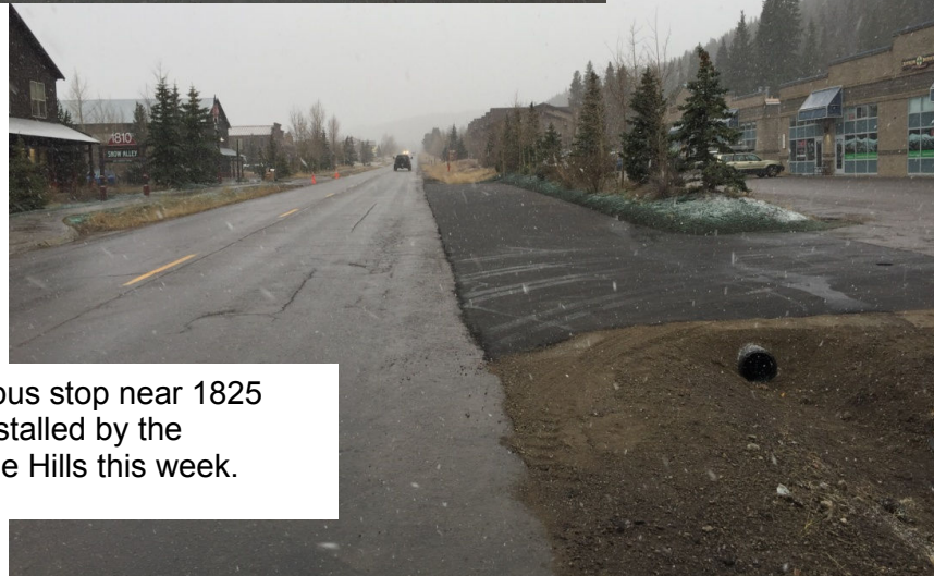
New lights are beginning to be installed by All Electric starting near the Airport Auto drive.
