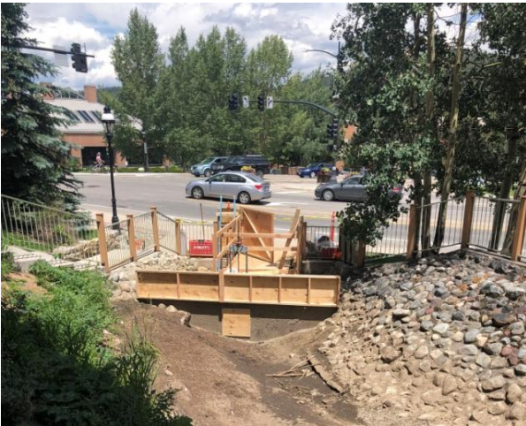
View of dewatered stream and staging area for culvert entry and debris removal.
