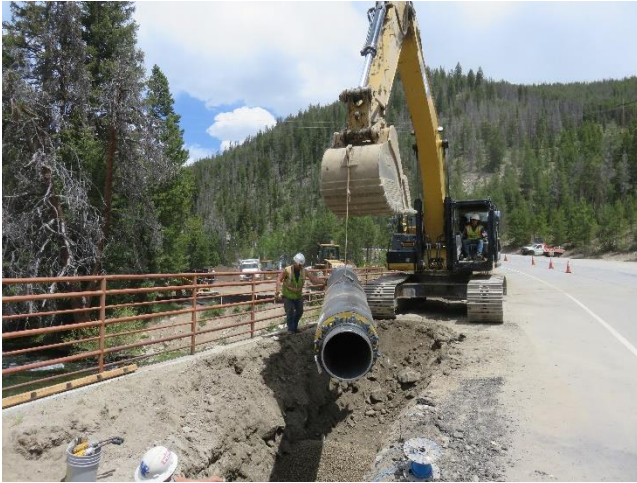
06/05/2018- Raw Water Pipe at Swan Mountain Road Blue River Crossing
